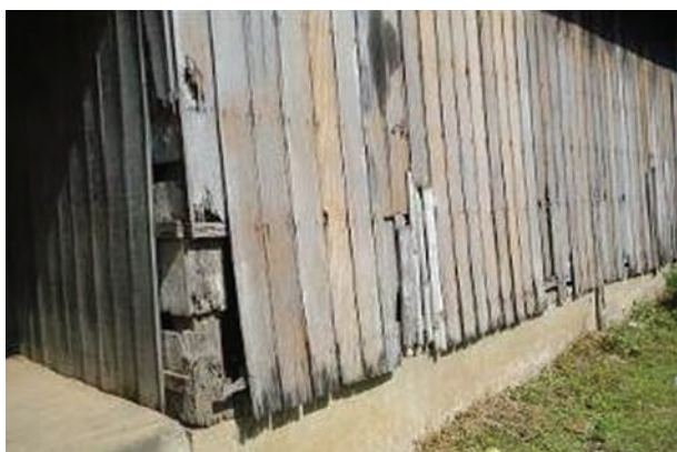
An unsafe structure which needs replacement. (Photo: PFERNA Team)
