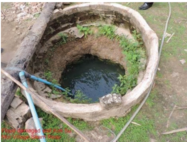
Flood Damaged well in Siem Riep (Photo: PFERNA Team)
